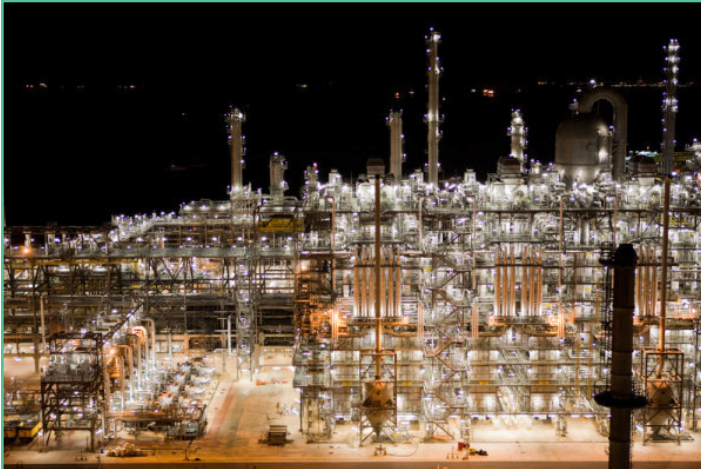
Figure 1: A Worldscale Shell Ethane Cracker in Singapore. Source: .Shell Flickr (CC-BY-NC-ND 2.0) https://creativecommons.org/licenses/by-nc-nd/2.0/
